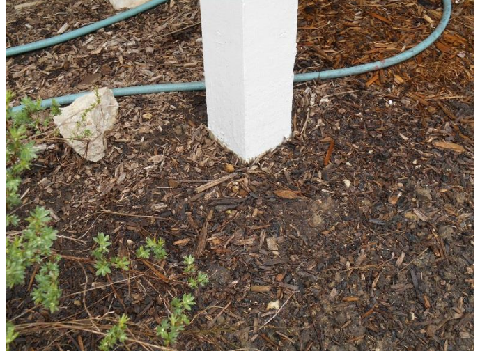
Support column below grade is subject to excessive moisture.
