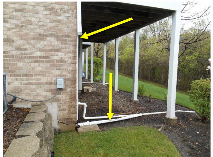
Disconnected downspout at unit 11006.
