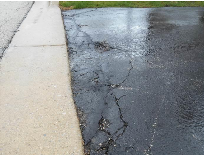
Typical asphalt deterioration.
