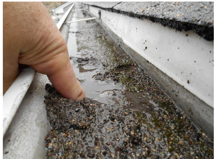
Shingle granular loss.
