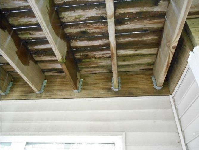
Inadequate balcony structural connection (i.e. no ledger board bolts).
