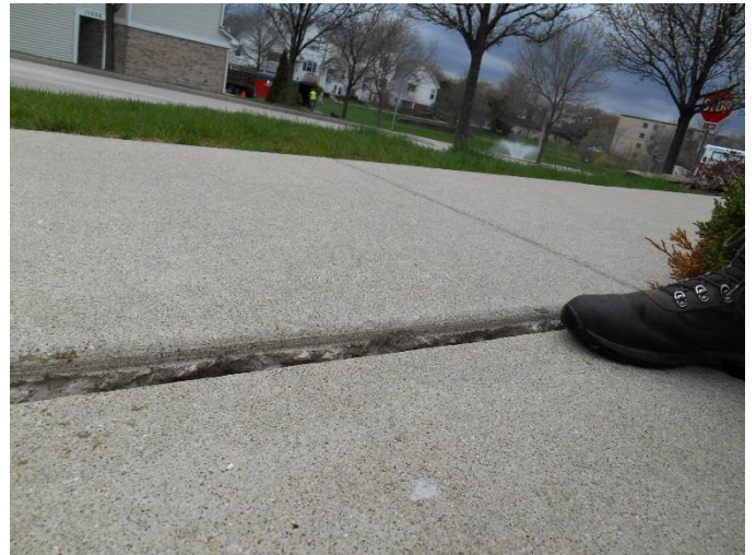
Trip hazard at the concrete entrance walkway to unit 11055.
