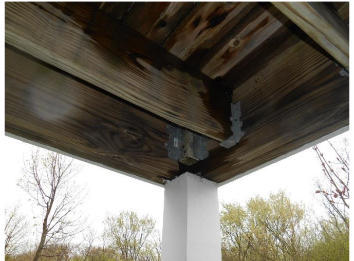
Inadequate balcony structural connection.
