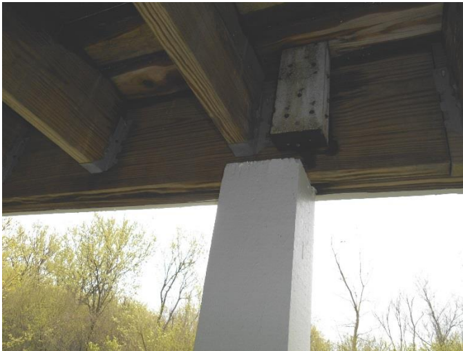
Inadequate balcony structural connection.
