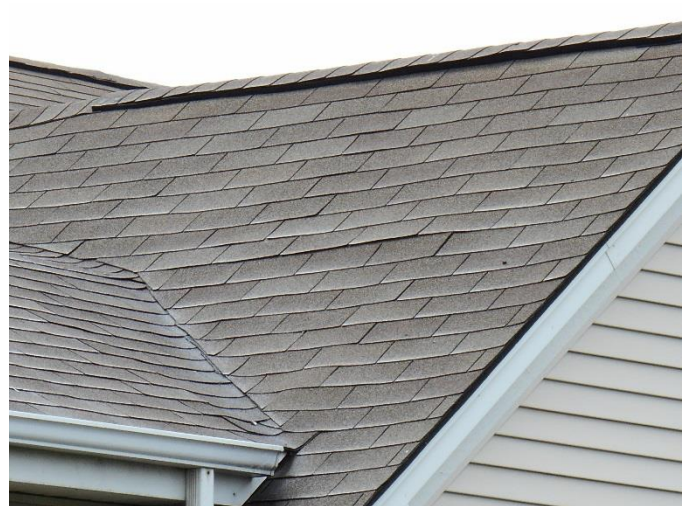
Shingles not laying properly.
