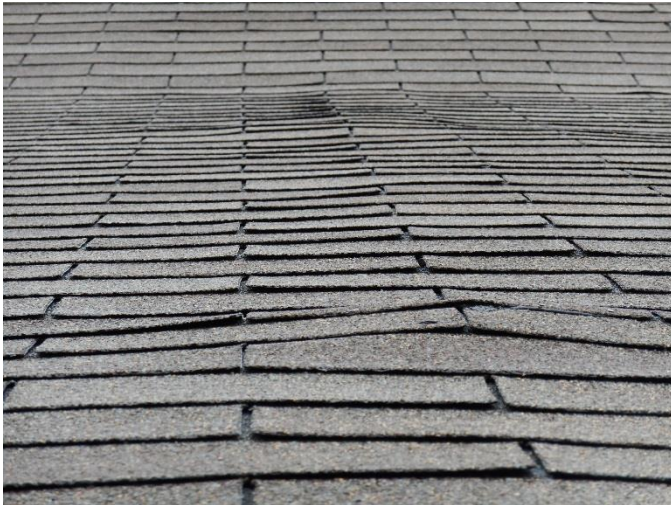
Uneven roof decking.
