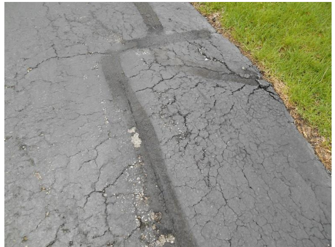
Typical asphalt deterioration.
