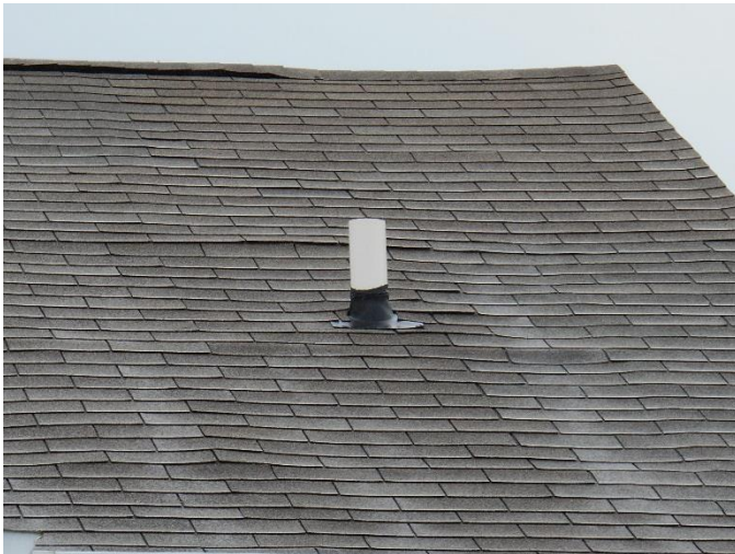
Shingles curling and not laying properly.
